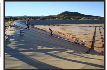
Floating Cover Reservoir
